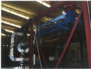
New 5MW isolator and new 5 MW klystron at modulator 3
