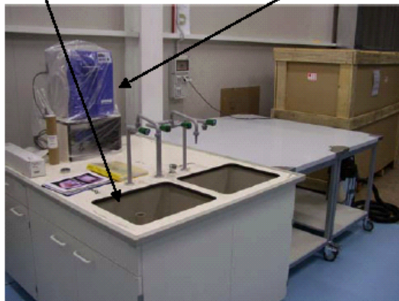
Washstand with high-purity water supply
